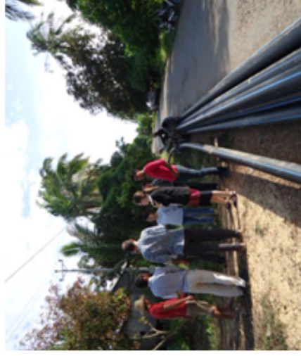
Main pipe installation and water service provider at Sambok commune Chher Borey district Kratie
